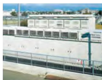
AC-DC converter equipment for Energy
